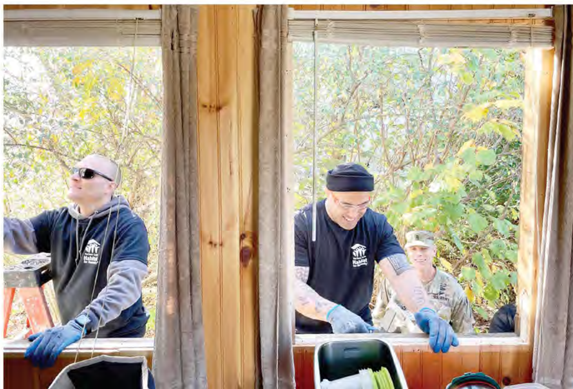
Pictured: The Northern Ocean Habitat for Humanity team works to replace windows at a home in Ocean County.
