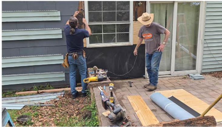
Starve Poverty team removed sections of siding and fascia to repair rotted wood and damaged framing before installing a new window and restoring the exterior of the home.
